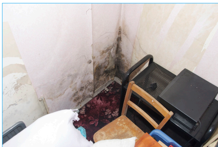
Figure 12: Mould growth and dampness.
