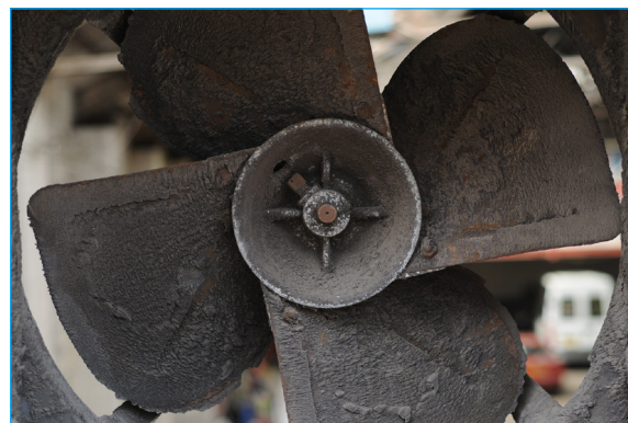
Figure 9: A dirty ventilation fan.
